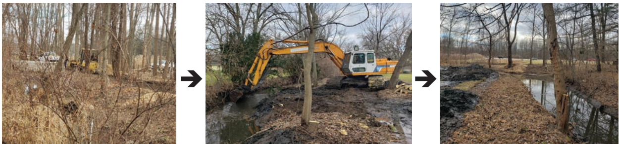
TASD removes debris that was causing water to collect and breed mosquitoes.
